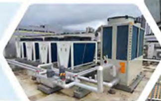
Integrated Air Handling Unit
